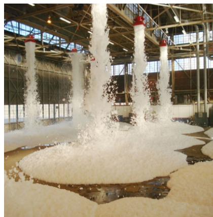
Foam System Discharge
