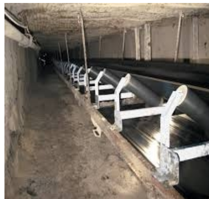
Typical Underground Belt
